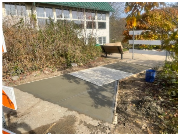
Figure 3. Pilot-scale deployment of CO 2 -sequestered ECC slabs (photo courtesy: Scott Spooner, City of Ann Arbor Parks and Recreation Services)
