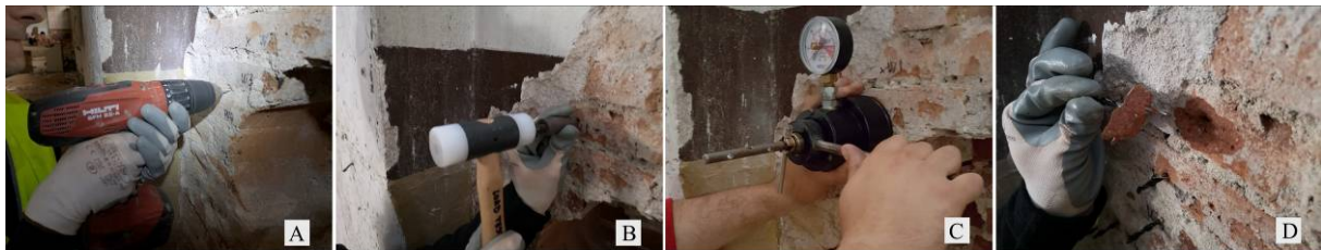
Figure 2: Helix Pull-out Test operation: (A) drilling the pilot hole, (B) hammering the tool until the helical tie is introduced in the pilot hole, (C) loading by turning the grip lever until failure, (D) failure in the brick.
