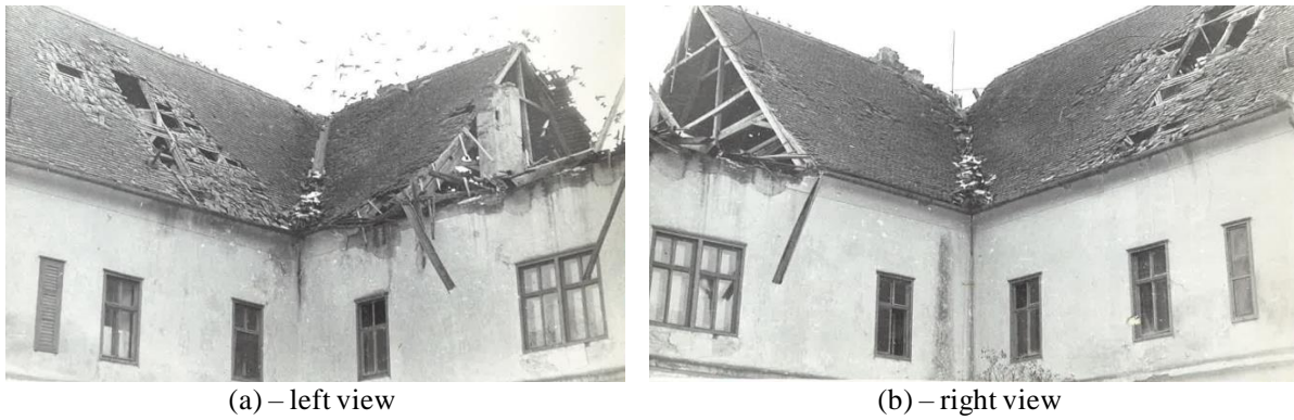
Figure 10: Failure mechanisms observed in the internal court of the case study building [19].
