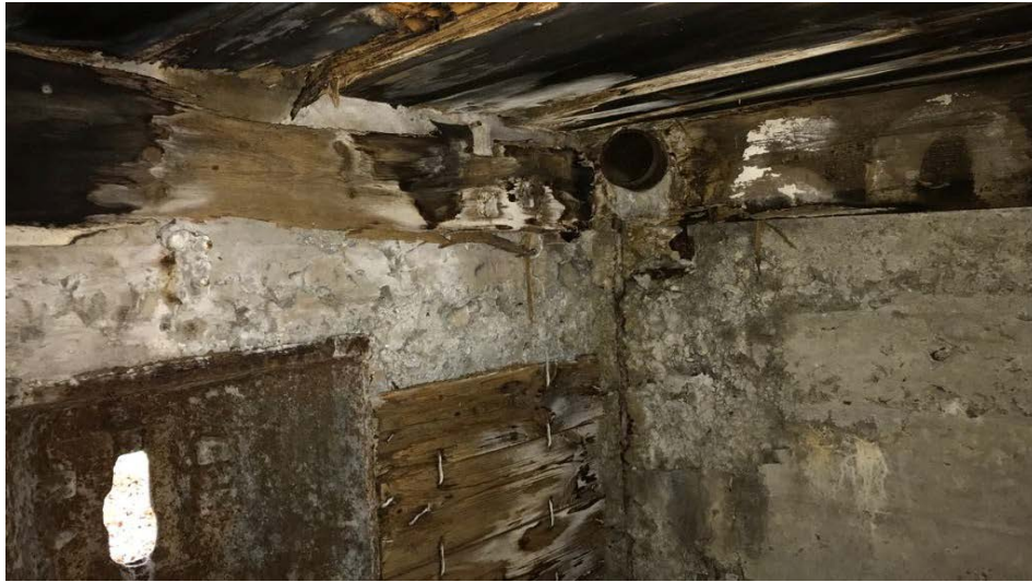
Figure 2. Residuum of internal timber cladding, poor quality of surface layer of concrete.
