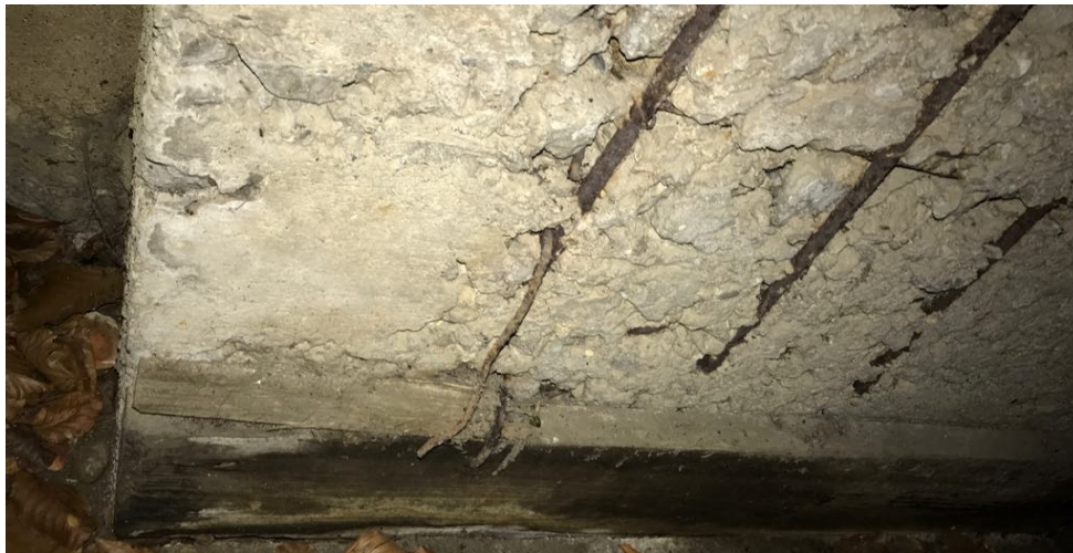
Figure 3. Insufficient compaction with uncovered steel reinforcement.
