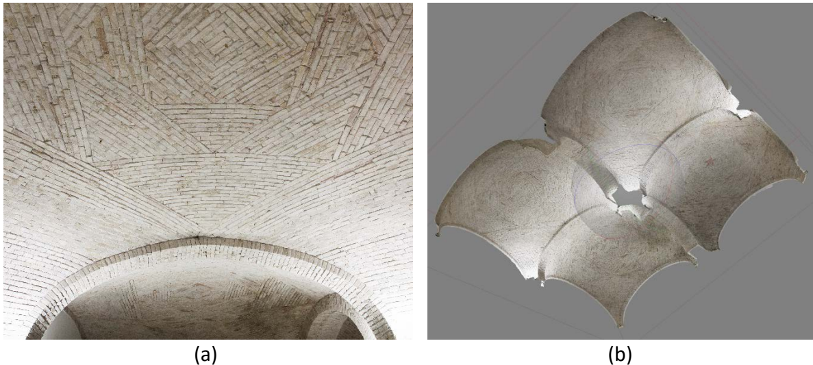
Figure 1. A typical lowered sail vault in Cagliari (a); geometry obtained by laser scanner survey (b).
