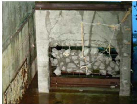
Figure 19.34: Cracked geometry of the wall after the experiment conducted in Arikawa et al. [ASI12].
