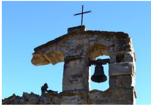
Figure 9: The damaged bell gable of San Paolo a Cortino (TE)
