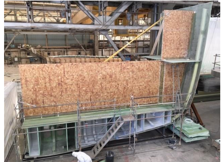
Demonstrator under construction at iXblue, La Ciotat, France showing laminated and sandwich construction
