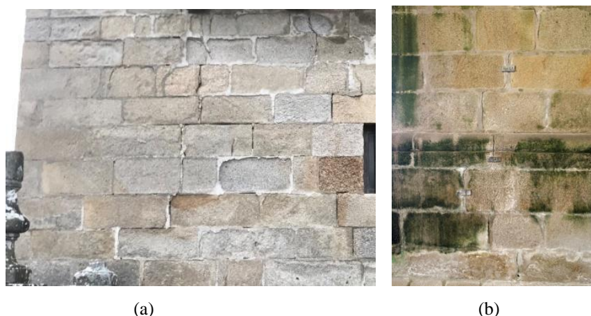
Figure 2: Cracks under the balcony of the tower in (a) external west facade and (b) internal east facade.
