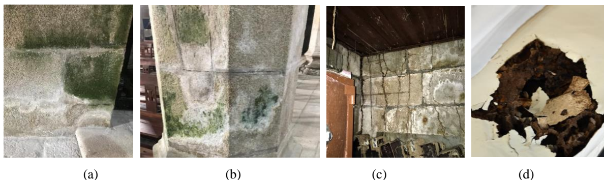
Figure 4: Algae observed on (a) interior walls and (b) column base; (c) termite infestation behind altar; (d) rot in altar
