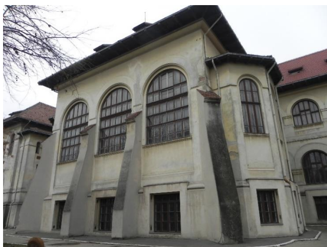
Figure 2: View of the back facade of the National Geological Museum (secondary wing)
