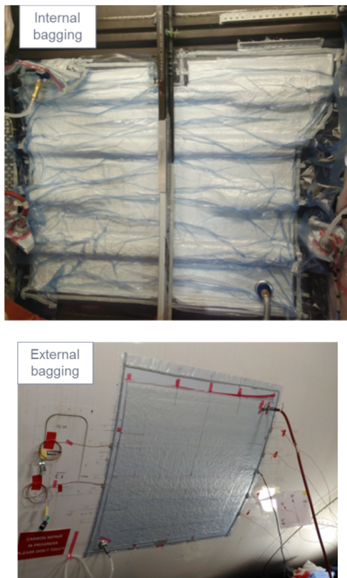
Figure 3 Internal and external bagging applied during the cure of a repair of a perforating damage in the fuselage skin
