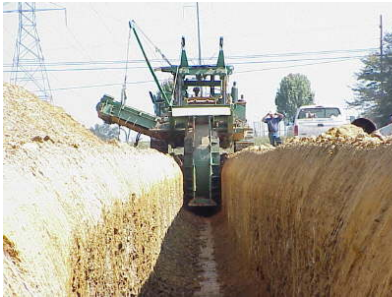
FIGURE 3.3-9 Pipeline Ditching (Source: Photo courtesy of U.S. Pipeline, Inc. Reproduced with permission.)
