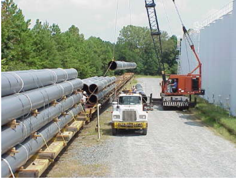
FIGURE 3.3-4 Pipe Segments Arriving at Rail Off-loading Area (Source: Photo courtesy of U.S. Pipeline, Inc. Reproduced with permission.)
