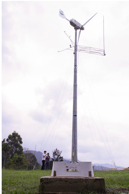
Figure 1: Wind turbine installed in EAFIT Llanogrande
