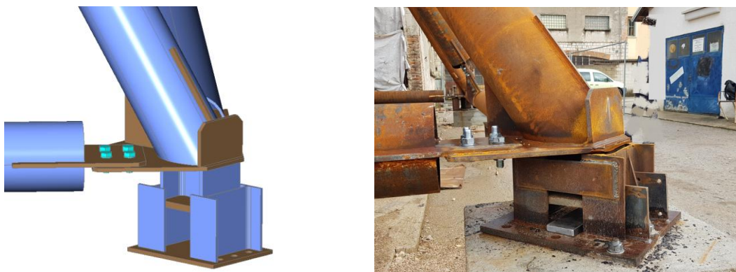
Figure 10: Software design of the steel bearing connection on the left and constructed on-site in the right
