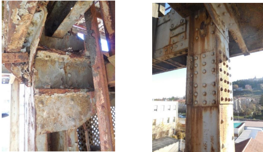
Figure 4: Coating condition – lower part of the structure on the left; upper part of the structure on the right
