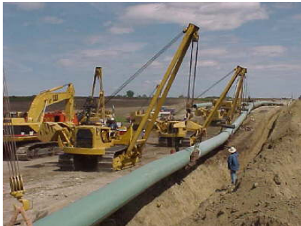
FIGURE 4.1-6 Crew Lowering a Pipeline into a Trench (Source: Photo courtesy of U.S. Pipeline, Inc. Reproduced with permission.)
