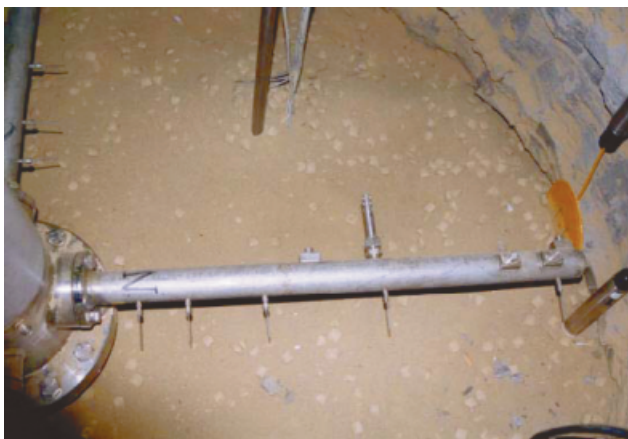
Fig. 1. Mixture of bentonite pellets and bentonite powder used as sealing material in an experimental shaft
