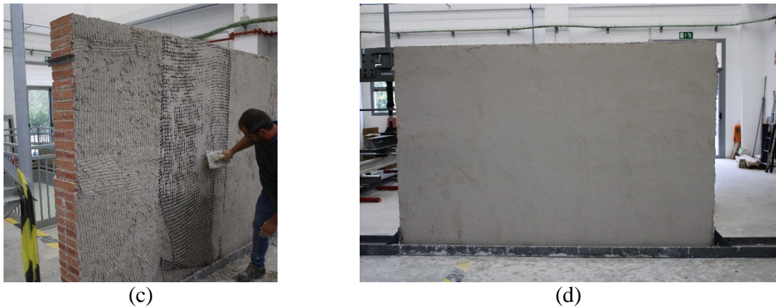
Figure 2. (a)- Injection the wider cracks. (b)- 5 mm thick cementitious laye applied on the outer face. (c)- Application of the glass fiber mesh. (d)- Reinforced masonry wall.
