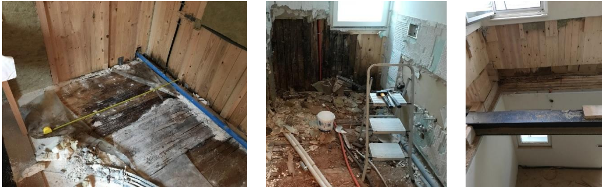
Figure 3. Pictures of damaged CLT slab and wall elements in hotel room.
