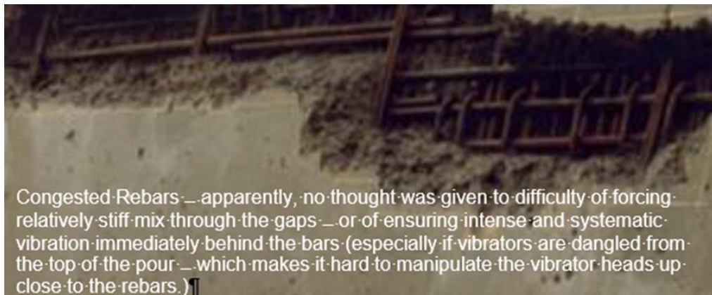
Figure 1. Close-up of Storebaelt Compaction Failure Showing Congested Reinforcement
