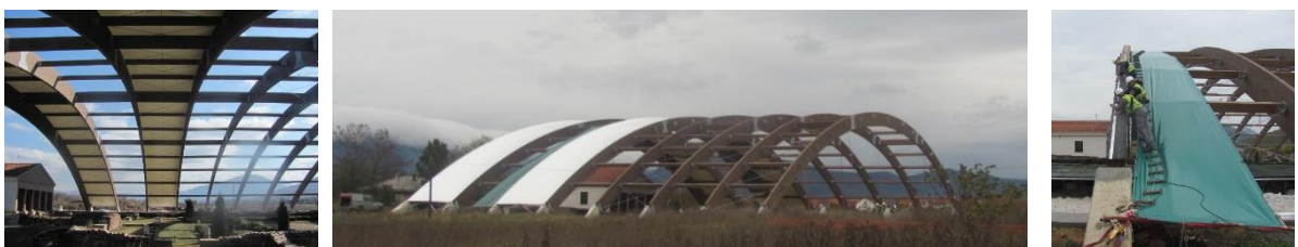
Figure 4: Scheme of alternating membrane panels installation (left, center), auxiliary membrane structure with marine ladders (right)
