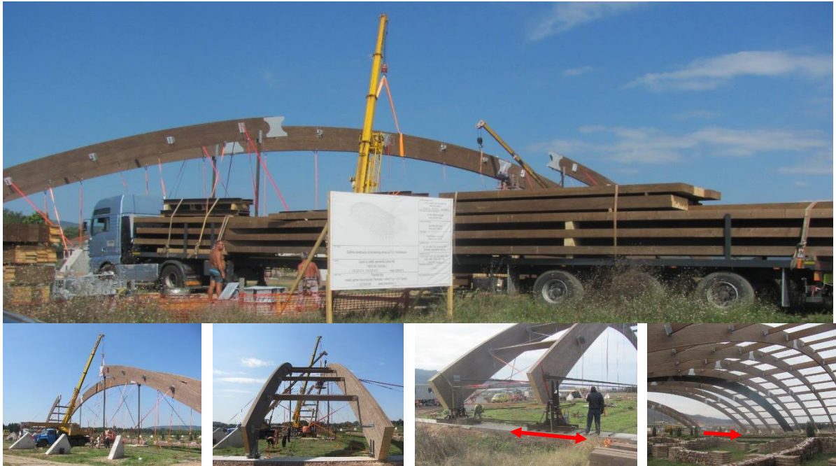
Figure 3: Special transportation of GLW elements on truck (top), preparation of first set of GLW arches (left, center left) and wagons under arch supports for moving and positioning of auto stable set (center right, right).
