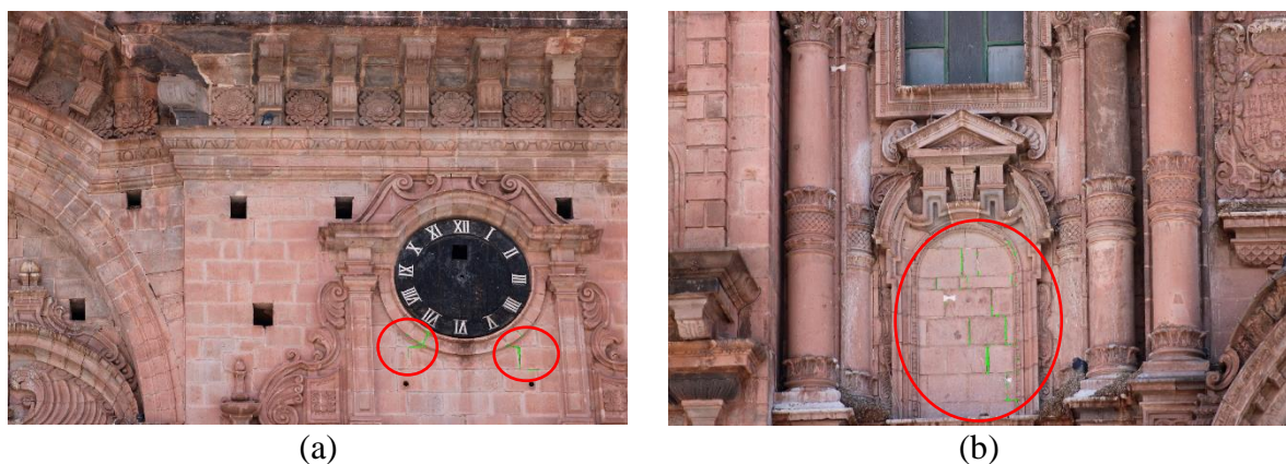
Figure 9: (a) Image 1 of the top part of the façade, (b) Image 2 of the middle part of the façade.
