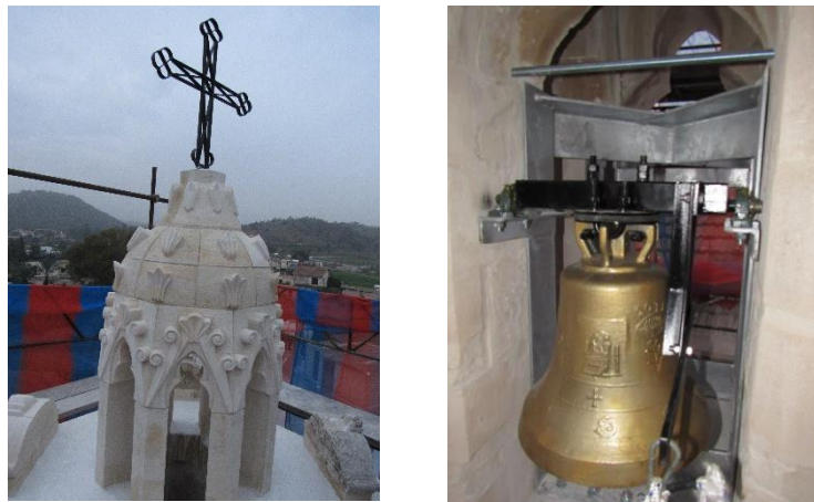
Figure 8: Restoration (left) and strengthening (right) of Saint John's bell tower in Psevdas (photos taken in December 2017)
