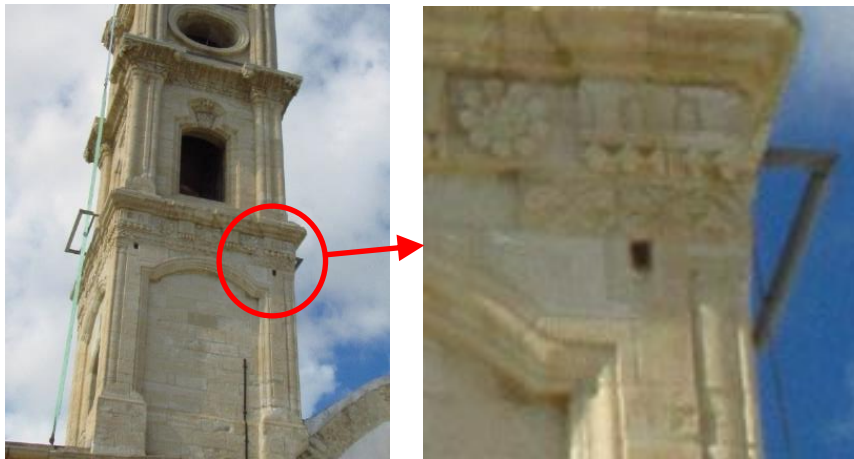
Figure 7: Bell tower of Saint John's church (left), Larnaca, where the anchorage of the cramps is visible (right)
