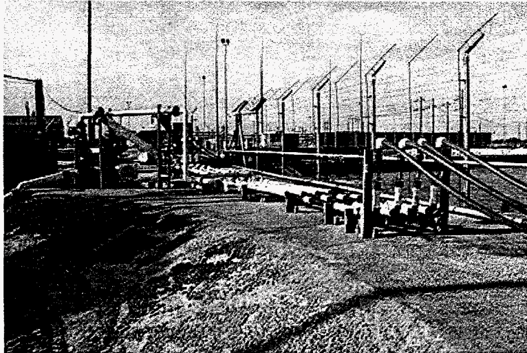
Figure 4. The flow-loop test manifold at Big Hill.
