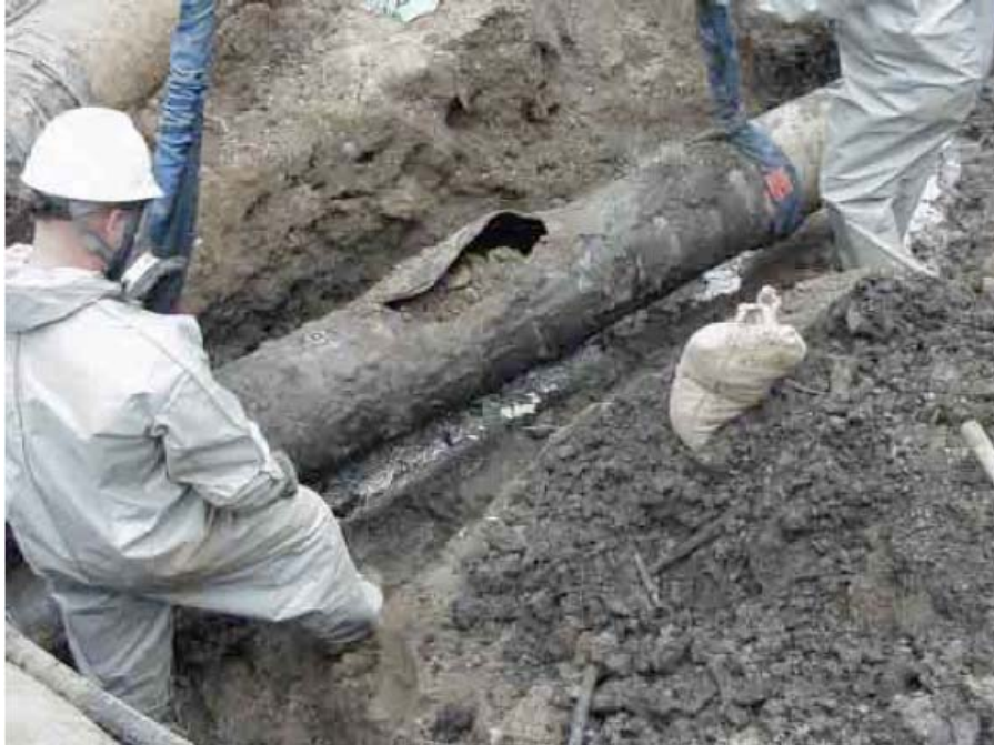
Figure 1.2: Actual rupture in the pipeline (NTSB, 2002)
