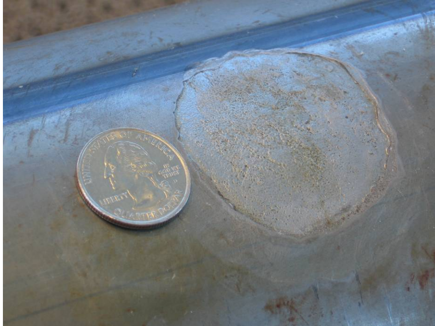
Figure 5.14: Top view of accelerated corrosion, 20% through thickness
