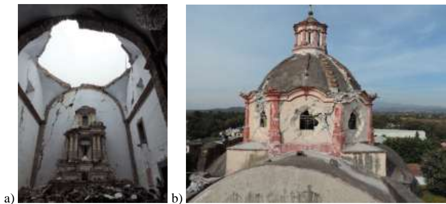
Figure 9: Damage to the main dome in temples in Morelos: a) Totolapan (sail vault); b) Zacualpan
