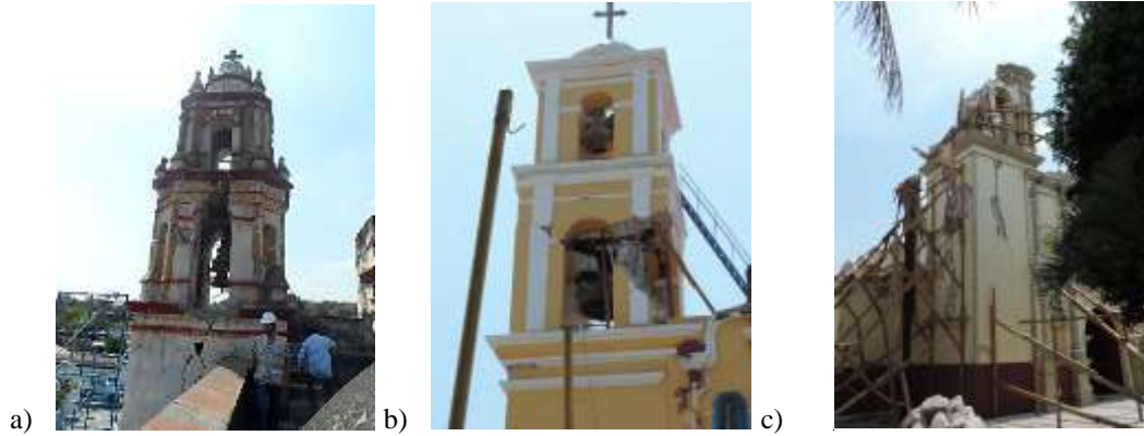
Figure 3: Damages patterns in bell towers: a) San Andrés de la Cal, Morelos; b) Santa Ana Jolalpan, Puebla c) Pilcaya, Puebla
