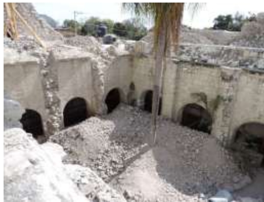
Figure 15: Damage to the cloister of the convent of Jantetelco, Morelos
