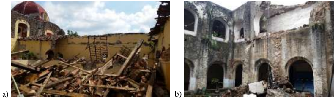
Figure 14: Damage to the upper cloister of Morelos convents: a) Juitepec; b) Totolapan
