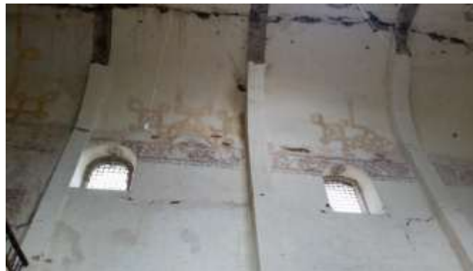
Figure 11: Horizontal wall cracks in the temple of Tlayacapan, Morelos
