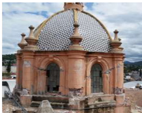
Figure 18: Damage in the dome of Huajuapán Cathedral, Oaxaca due to interventions before to the 2017 earthquakes
