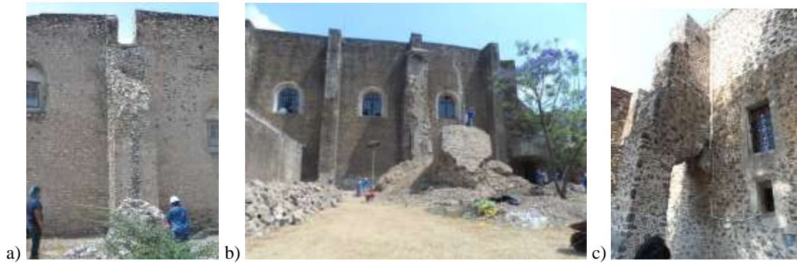
Figure 12: Typical damage to butresses in Morelos: a) Tlayecac; b) Tlayacapan and c) Totolapan
