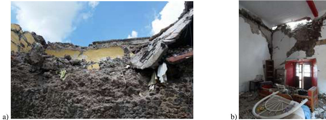
Figure 19: Wall collapses due to interventions with concrete slabs in the convent of Jiutepec, Morelos: a) Slab supported directly on the wall; b) Beams supported on the walls
