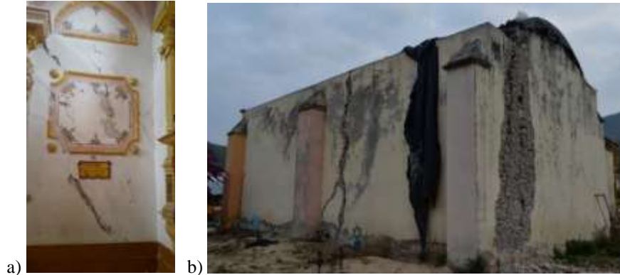
Figure 10: Damage in side walls: a) El Calvario temple, Huajuapán, Oaxaca; b) Ayoxutla, Puebla
