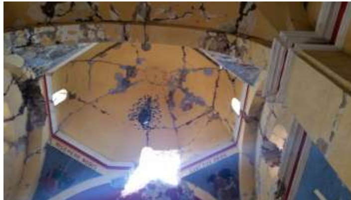
Figure 8: Radial and meridian cracks in the dome of the Jiutepec temple, Morelos
