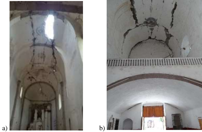
Figure 7: Damage in vaults: a) Tlayacapan, Morelos and; b) Tlaquiltenango, Morelos
