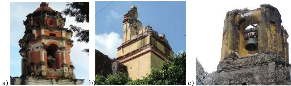
Figure 4: Damage to facades of temples in Morelos: a) Hueyapan; b) Jiutepec; c) Ocuituco
