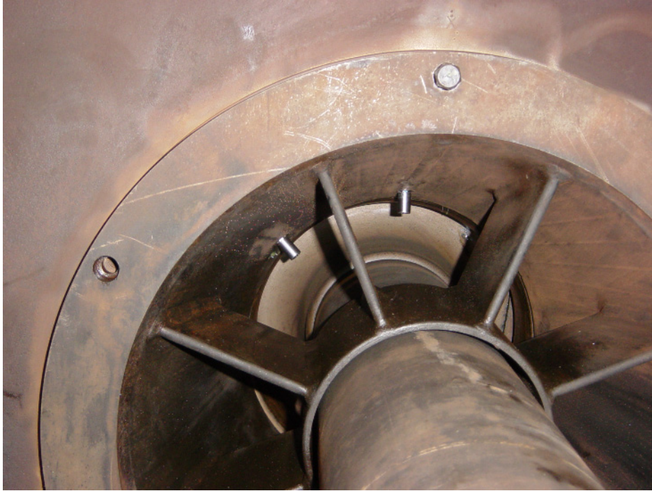
Figure 4-27. Surge Detection Probes Installed in Front of Field Site Compressor Impeller.
