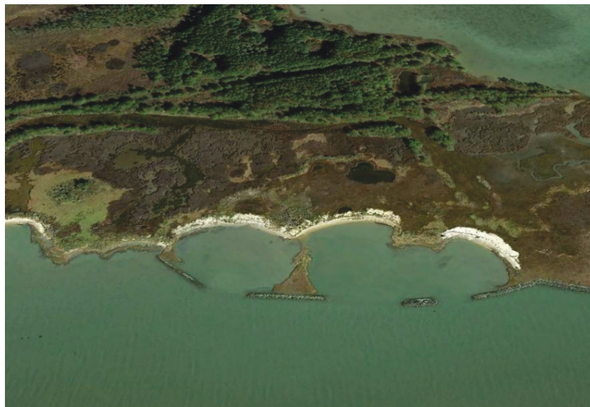
Figure 6. Barren Island segmented breakwaters designed and constructed to promote natural tidal flows to stabilize coastal marsh habitat (Images sourced from Google, DigitalGlobe 2017).
