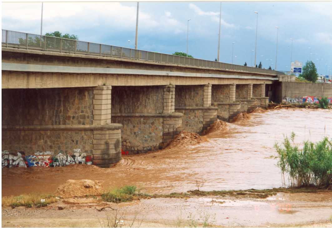
Figure 9.41 - Llobregat river flood of 9 th June 2000. View of Sant Boi bridge. Upstream
