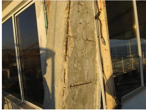
Figure 6: Actual condition of some structural elements [11]
