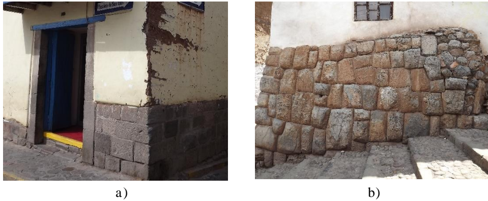
Figure 3: Main foundation typologies: the most recent stone foundations (a) and the ancient Inca foundations (b).
