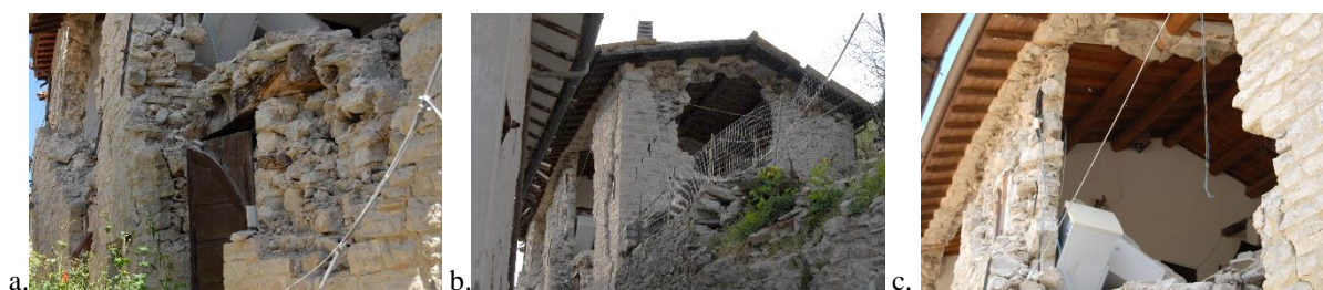
Figure 3: Examples of poor seismic behaviour in a strengthened masonry building, CSN: a) Not effective tie rods on bad quality masonry; b) overturning of last storey and c) of internal bearing walls due to r.c. curbs and to excess of stiffness and weight of reinforced timber roof
