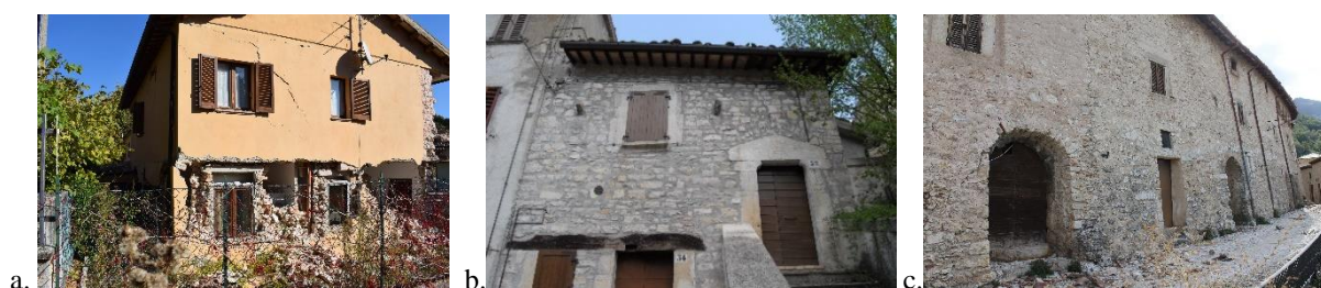
Figure 5: a) Class A building: poor masonry quality and floors replaced with rigid ones (MCC); b) C class building: random layout limestone masonry reinforced by deep repointing with cementitious mortar (CSN); c) D class building: random layout limestone masonry reinforced by grout injections and r.c. jacketing (internal side) (CMP)
