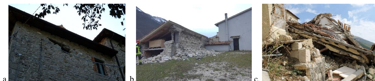
Figure 4: Examples of damage due to rigid roofs: a) Slip of the roof and horizontal arch (VZZ); b) Masonry leaves separation and local overturning (CSN); c) Total collapse due to crumbling of masonry (CMP)
