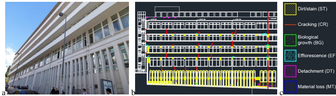
Figure 2: a) Part of the NW1 façade (Authors, n.d.), b) Defects marked on the NW1 façade (drawing taken from Istanbul University - Construction and Technical Department and adapted by authors), c) Main type of defects legend.
