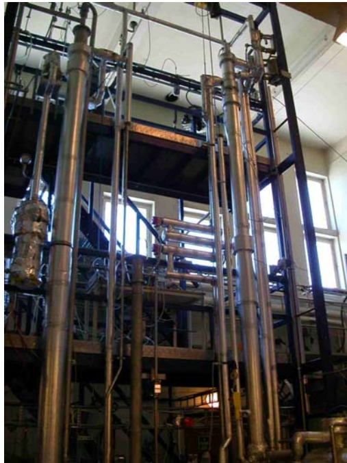
Figure 2 SINTEF Low Pressure Pilot Unit – Upper Half
