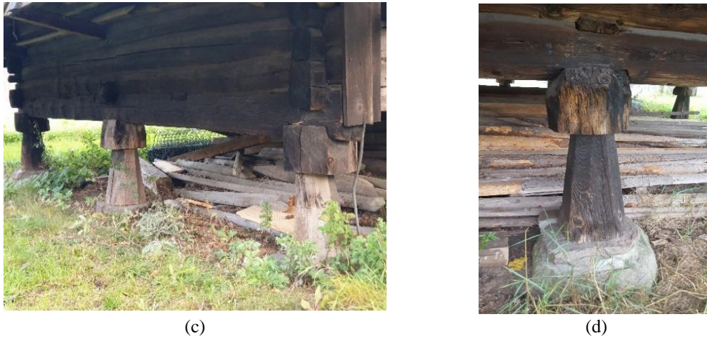
Figure 6: (a) Fadum Storehouse view, (b) Structural detail inside the coating, (c) Timber short columns under the building, (d) detail of the simply connected timber column
