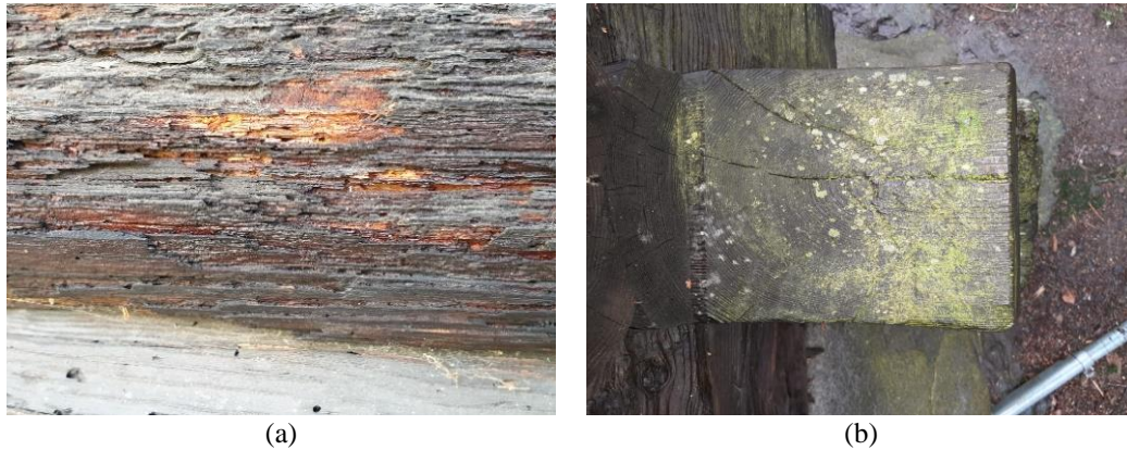
Figure 5: Biological defects in Heierstad Loft
