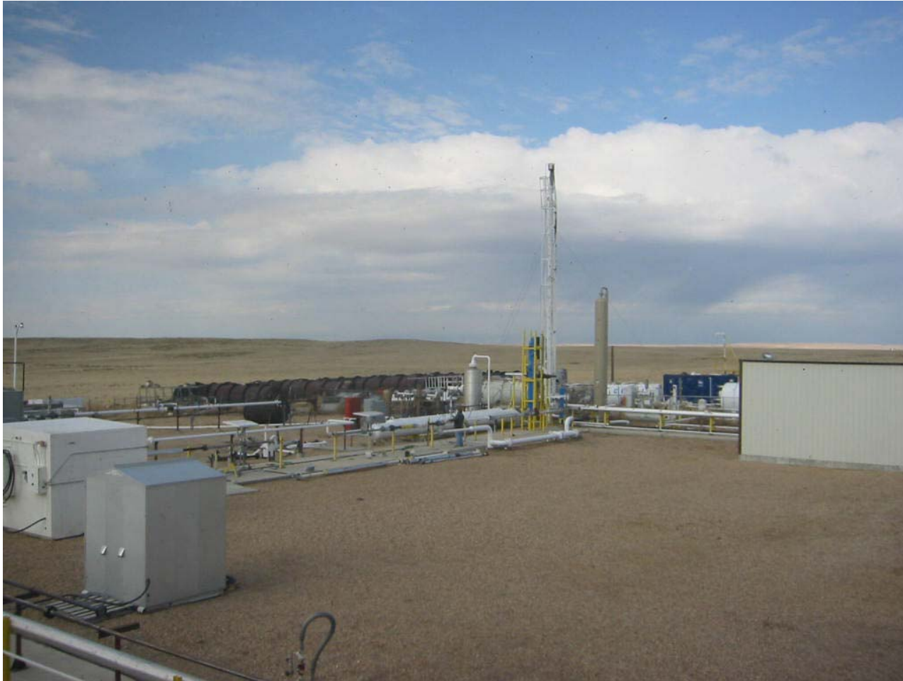
Figure 45 CEESI High Pressure Gas Test Facility
