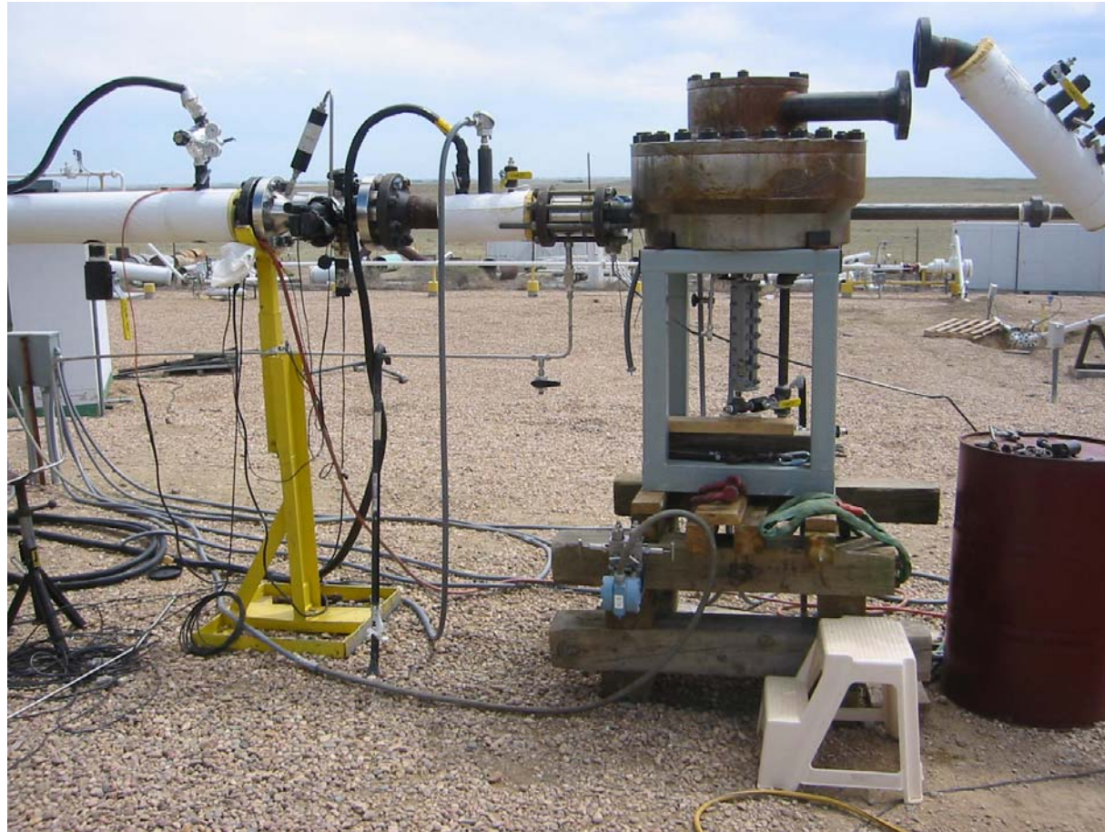
Figure 48 Multiple Nozzle Integral Separator and Upstream Piping Installed for Testing
