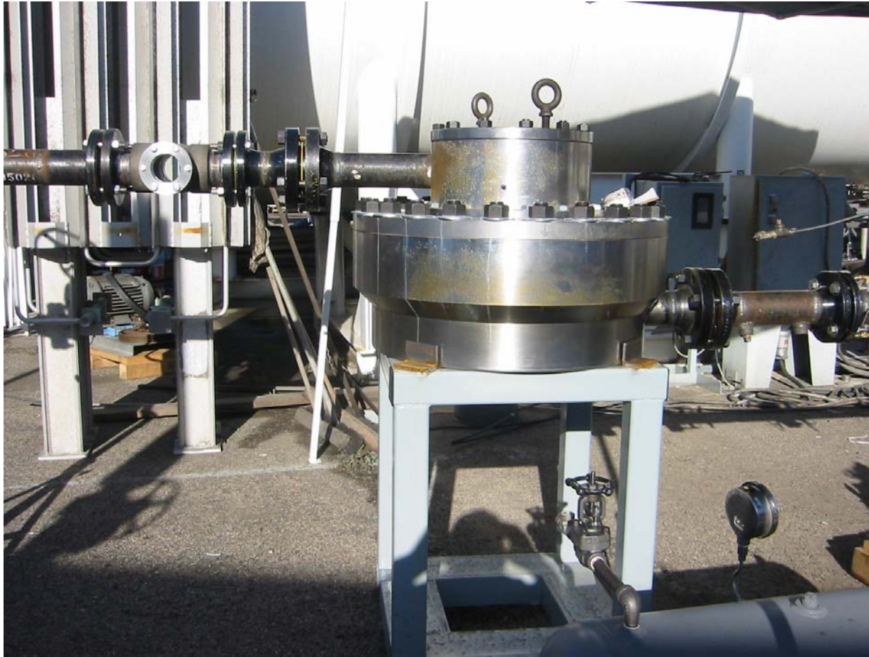
Figure 41 Separator on Test Stand in Nitrogen-Water Test System
