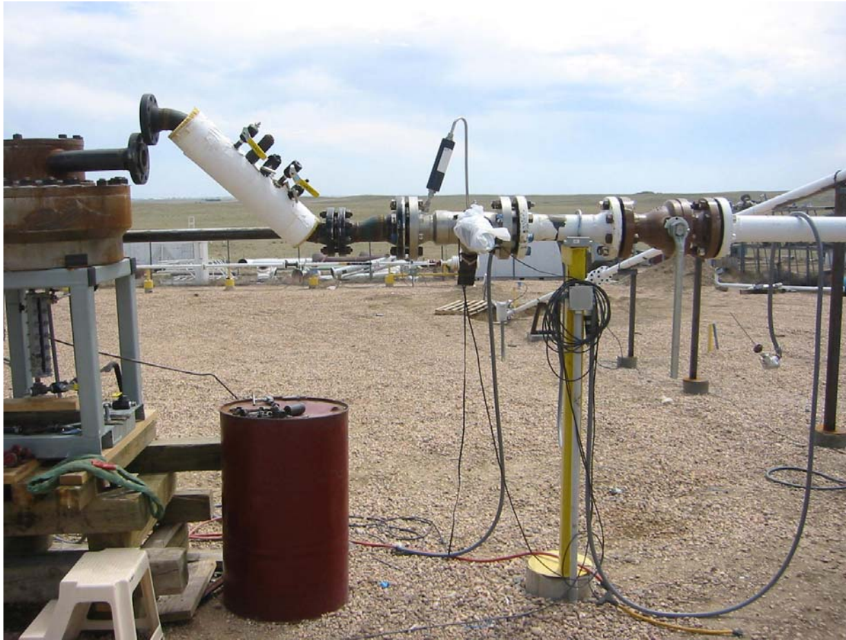
Figure 49 Downstream Piping from Integral Separator
