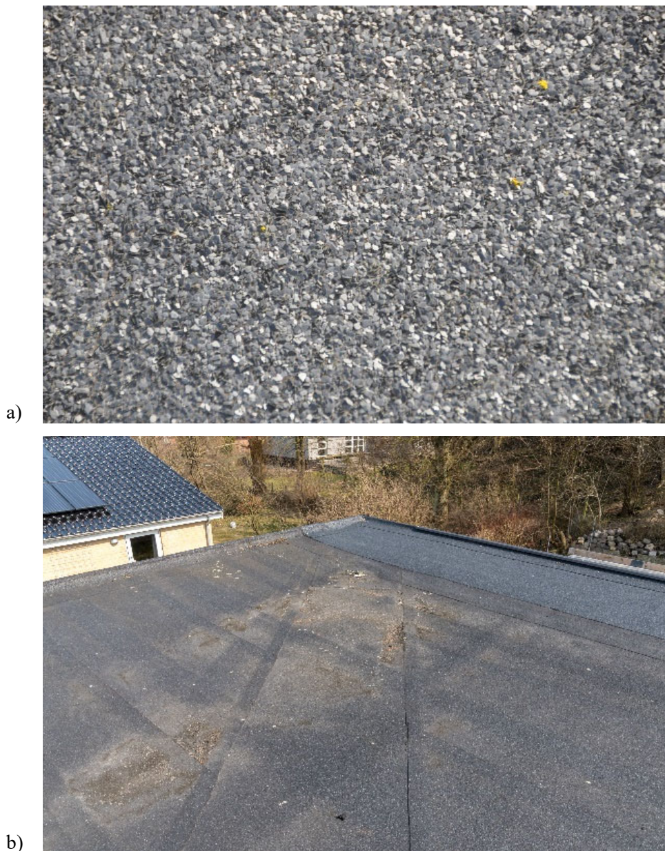
Figure 2. Roof condition at different points. a) Condition of slate is generally good as shown, b) roof valley in equal conditions as other parts of roof membrane.
