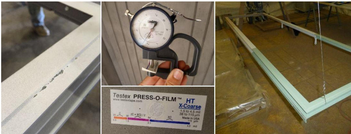
Figure 4. Steel frame blasting and surface profile measurement (left and center); coating mockup (right).
