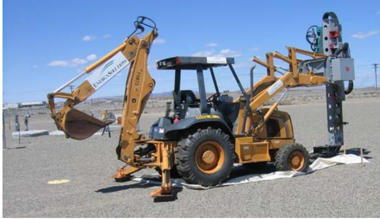
Figure 4.2. Hydraulic Hammer Used to Install Instruments in the T Tank Farm (Photo taken in the summer of 2006)
