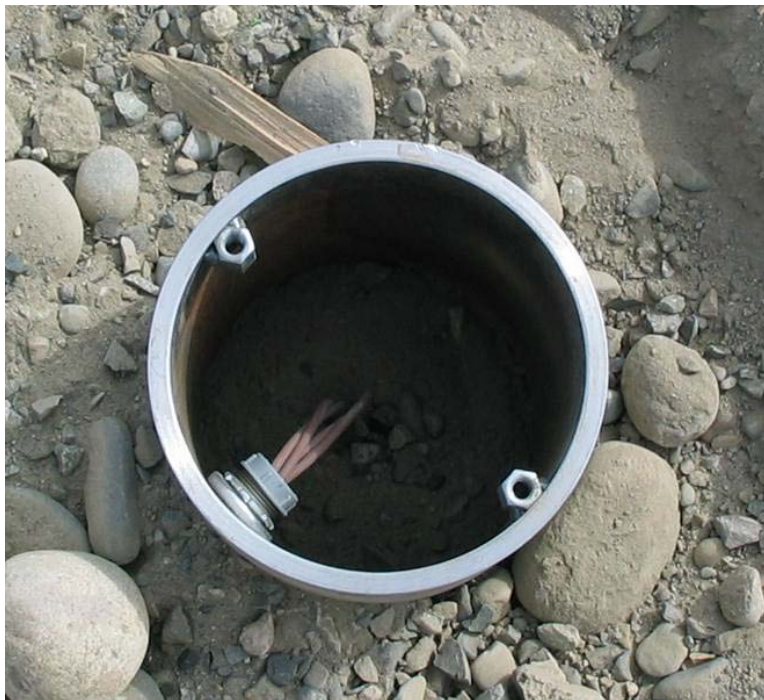
Figure 4.12. Protective Casing Over the HDU Location at Instrument Nest TB (Photo taken in the summer of 2006)
