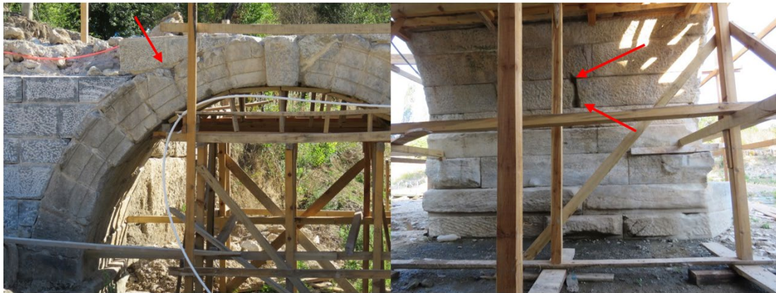
Figure 4. Some damages on joints
