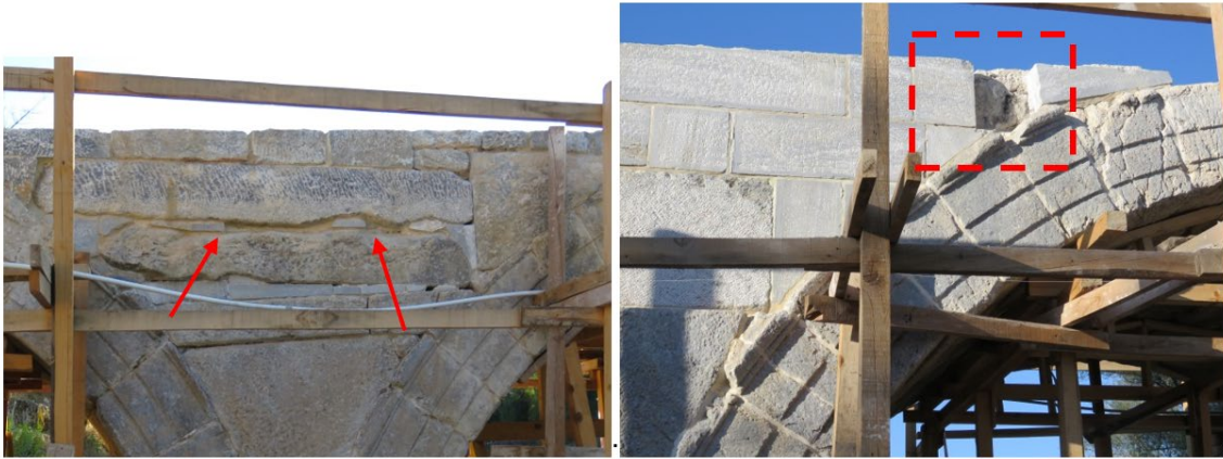
Figure 3. Material losses and joint damages
