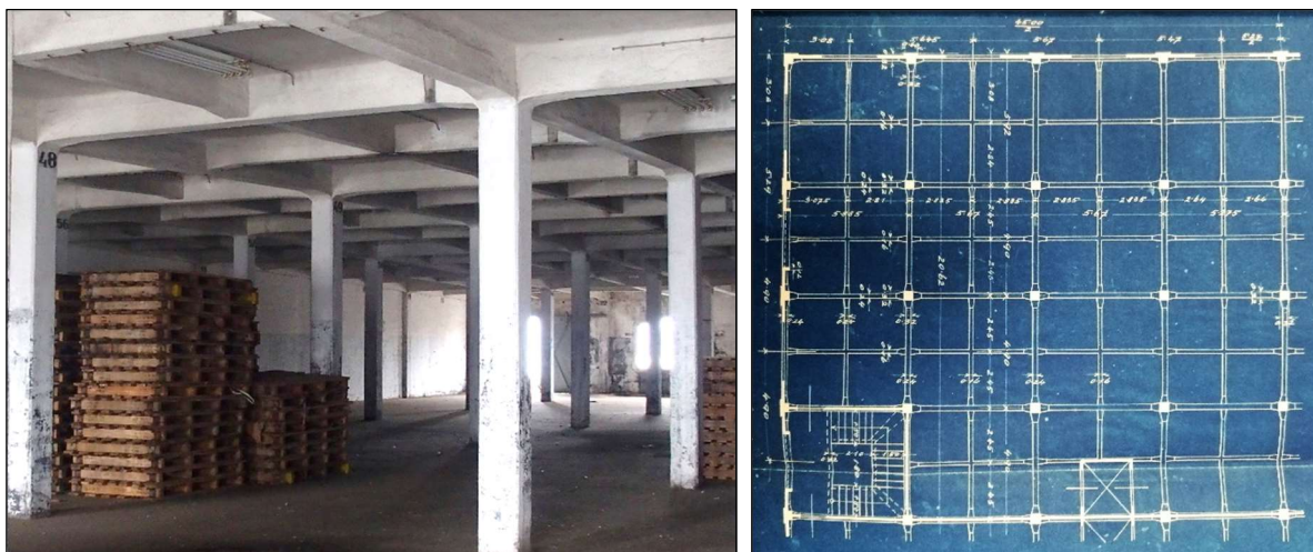
Figure 5: Layout of the basic column grid (5,6x4,9 m), primary and secondary beams on the 3 rd floor [5]
