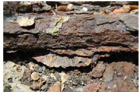
(g) Rebar so corroded that has a thick oxide layer in the surface
