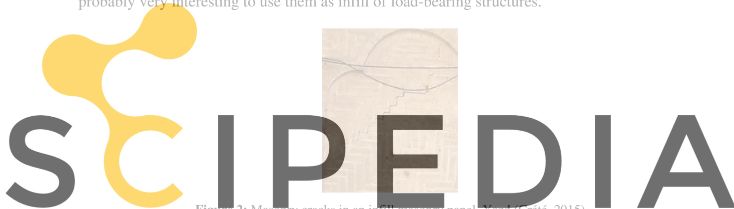
Figure 2: Masonry cracks in an infill masonry panel, Yazd (Crété, 2015)
