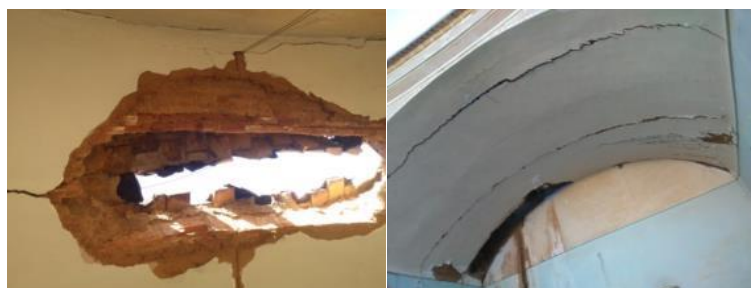
Figure 4: Baked bricks rows in an adobe vault and the creation of sectional cracks, the example of Shamsaei house, Yazd (Crété, 2015)
