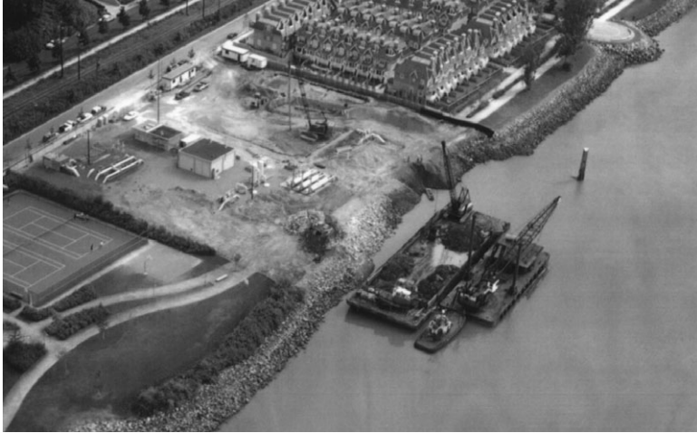
25.4 Ground densification using vibro-replacement at a river bank in Vancouver, British Columbia, Canada, to reduce the risk of liquefaction-induced lateral ground displacements (Wijewickreme et al. , 2005).
