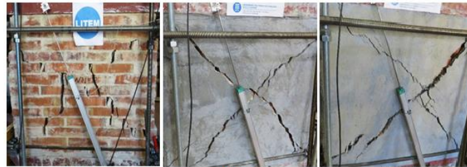
Figure 3. Specimen failures: WN, WNM, and WG
