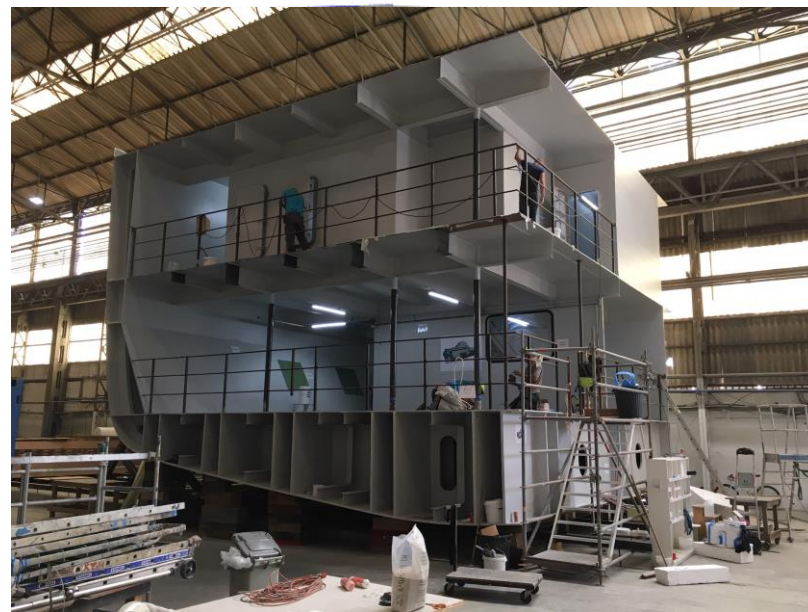
Demonstrator: Engine room and other above accommodation spaces. (Approx.: 11m x 11m x 8.6m)
