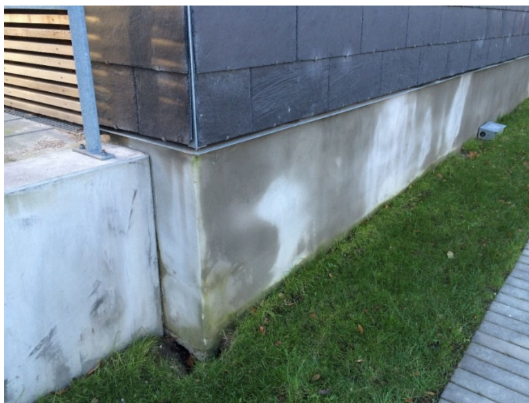
Figure 1. Wetting of a concrete foundation revealing that salty liquid has been released from MgO boards in the above lightweight external wall. Photo: Tommy Bunch-Nielsen.
