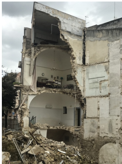
Figure 1. Partial collapse of a building after the demolition of the adjacent building (Oct 2019, Andria, Italy).
