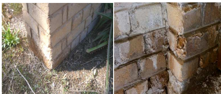
Figure 8. Degradation observed in the north region (humid pathology).
