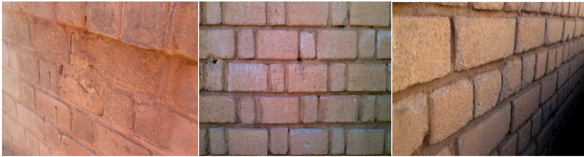
Figure 10. Direct impact of the mechanical action of the wind.
