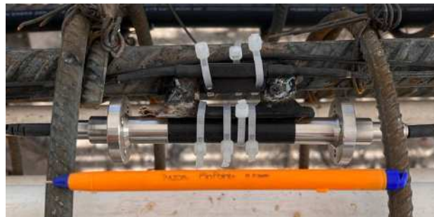
Figure 13: Strain and temperature FBG instrumentation
