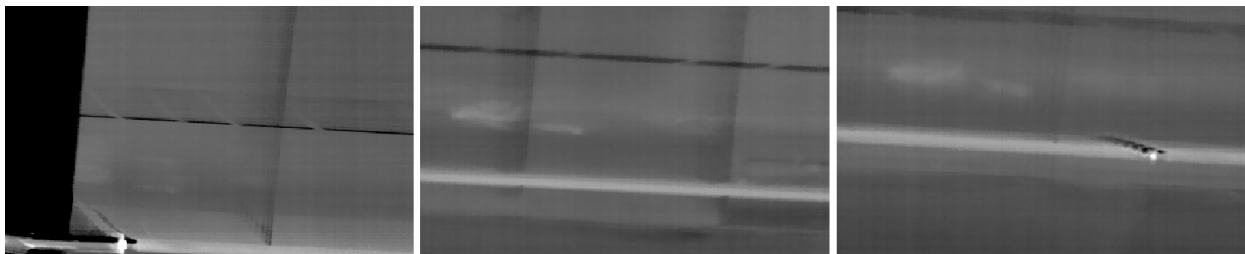
Figure 6. Sequence of thermographic images on Valle facilities.
